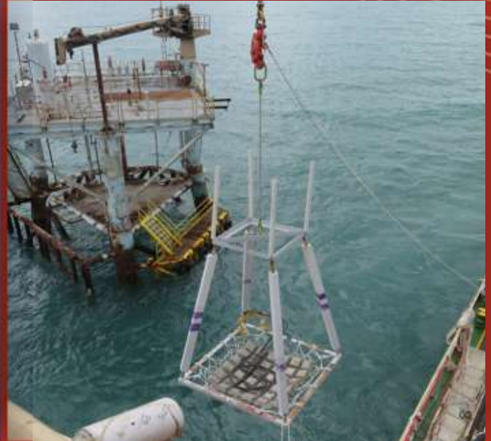
CP ANODE POD DEPLOYMENT PROCESS
